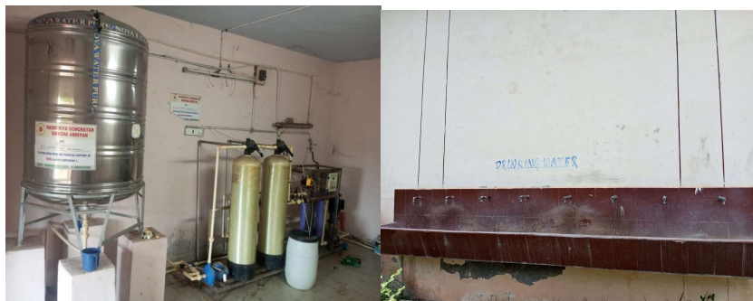
RO plant drinking water for students
