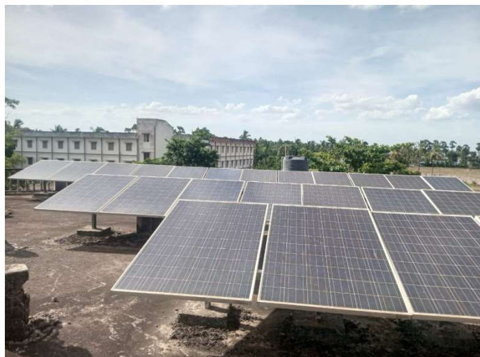
Solar Panels on the roof top
